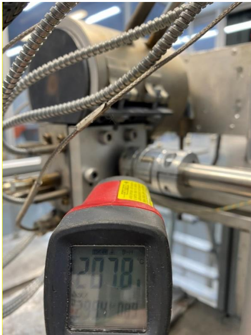
Fig. 4: Measurement of the ambient temperature at the gear, 207°C are measured.
